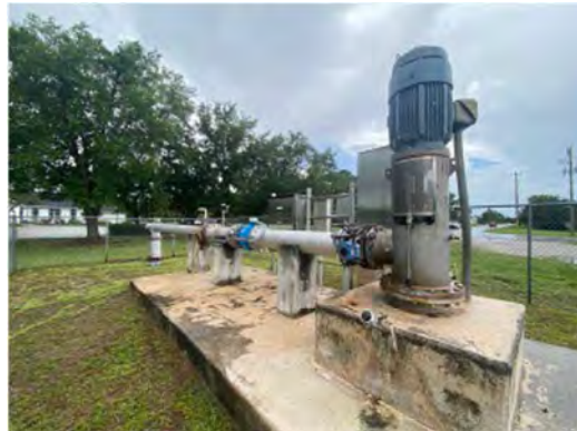
SLWSD Floridan Aquifer Well No. 1
