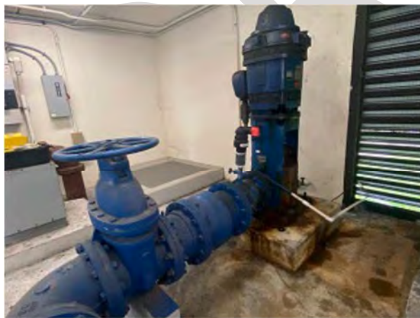
SLWSD ROWTP Transfer Pump
