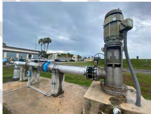
SLWSD Floridan Aquifer Well No. 3
