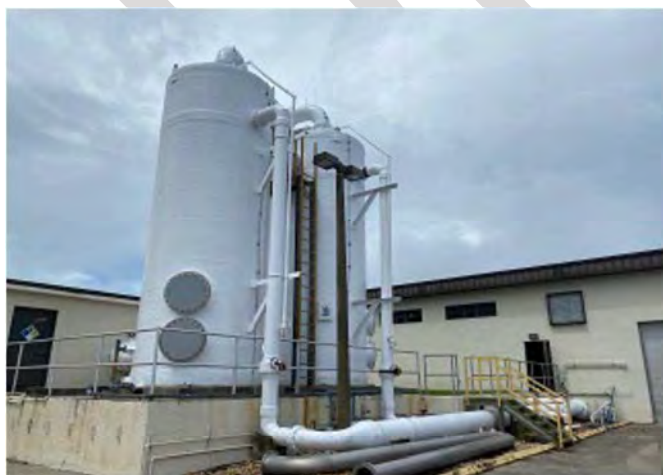
FIGURE 12. Degasifier Odor Control Unit
