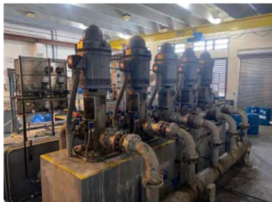
ROWTP High Pressure Feed Pumps
