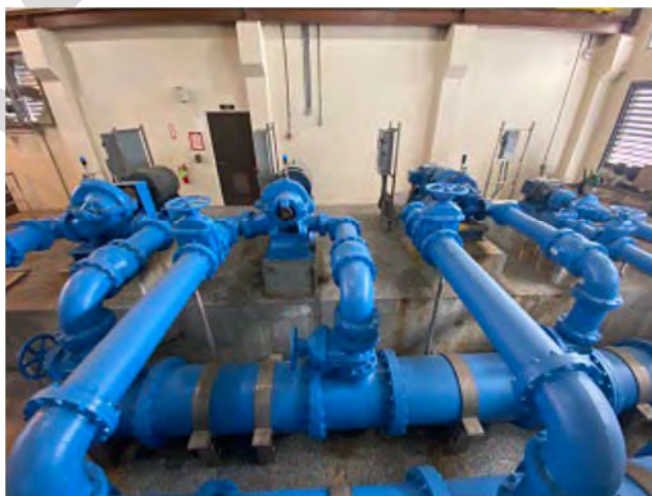
ROWTP High Service Pumps Set A (upgraded 2019)
