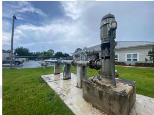
SLWSD Floridan Aquifer Well No. 2
