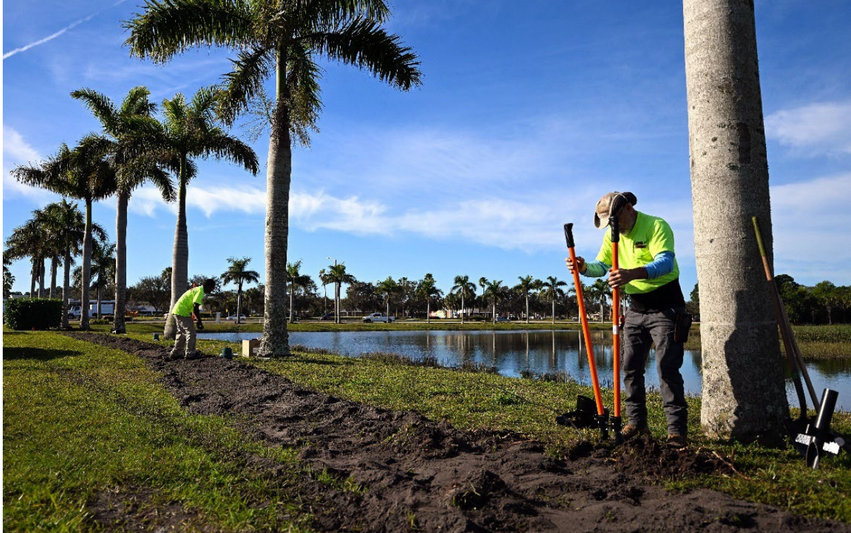
PORT ST. LUCIE, Fla -- Landscape contractors working with St. Lucie West Services District (SLWSD) excavate trenches Jan. 27, 2025; to install underground electrical cables to power up the palm tree lights around Lake Harvey. The artificial lake is located between St. Lucie West Boulevard and NW Cashmere boulevard. SLWSD has led a multi-phase project to improve the lake's ecology and make it a community landmark. (Photo by Anderson Bomjardim)
