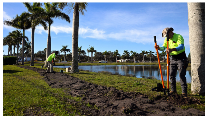
Landscape contractors working with St. Lucie West Services District (SLWSD) excavate trenches Jan. 27, 2025; to install underground electrical cables to power up the palm tree lights around Lake Harvey.
